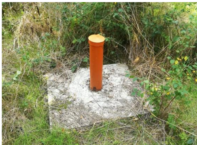
Installation externe ©NL
